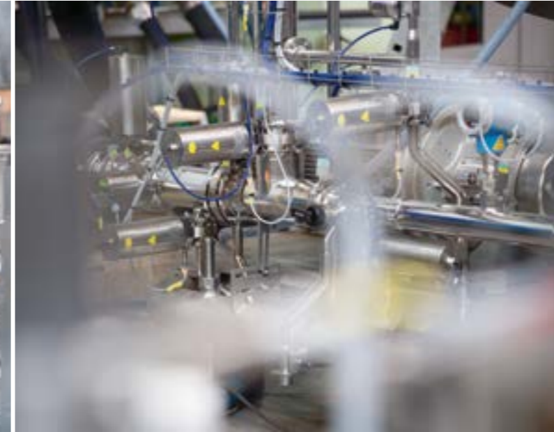
Digital software modules control the plant components.
